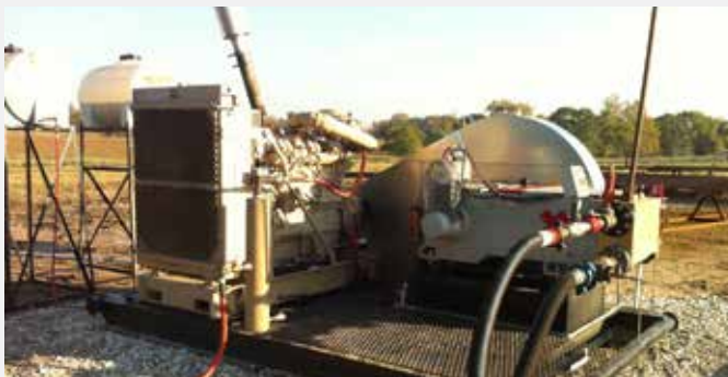
Tally's permanent unit with Cummins natural gas engine.
